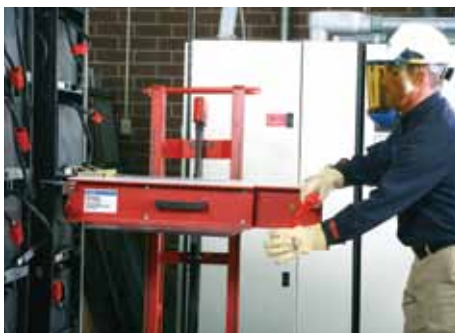
Larger UPS models require on-site preventive maintenance visits for optimal performance
